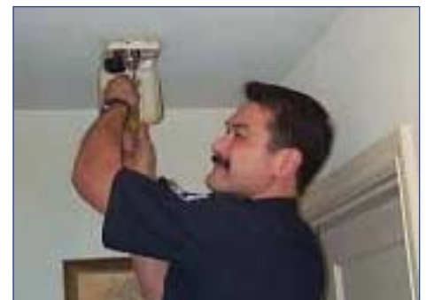
Photo courtesy of www.ci.seattle.wa.us/fire/pubEd/smokealarms/smokeAlarms.htm
